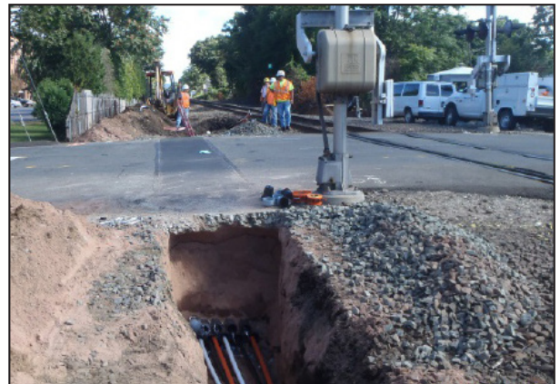
Pulling innerduct and cable below the grade crossing on Parker Street in Wallingford
